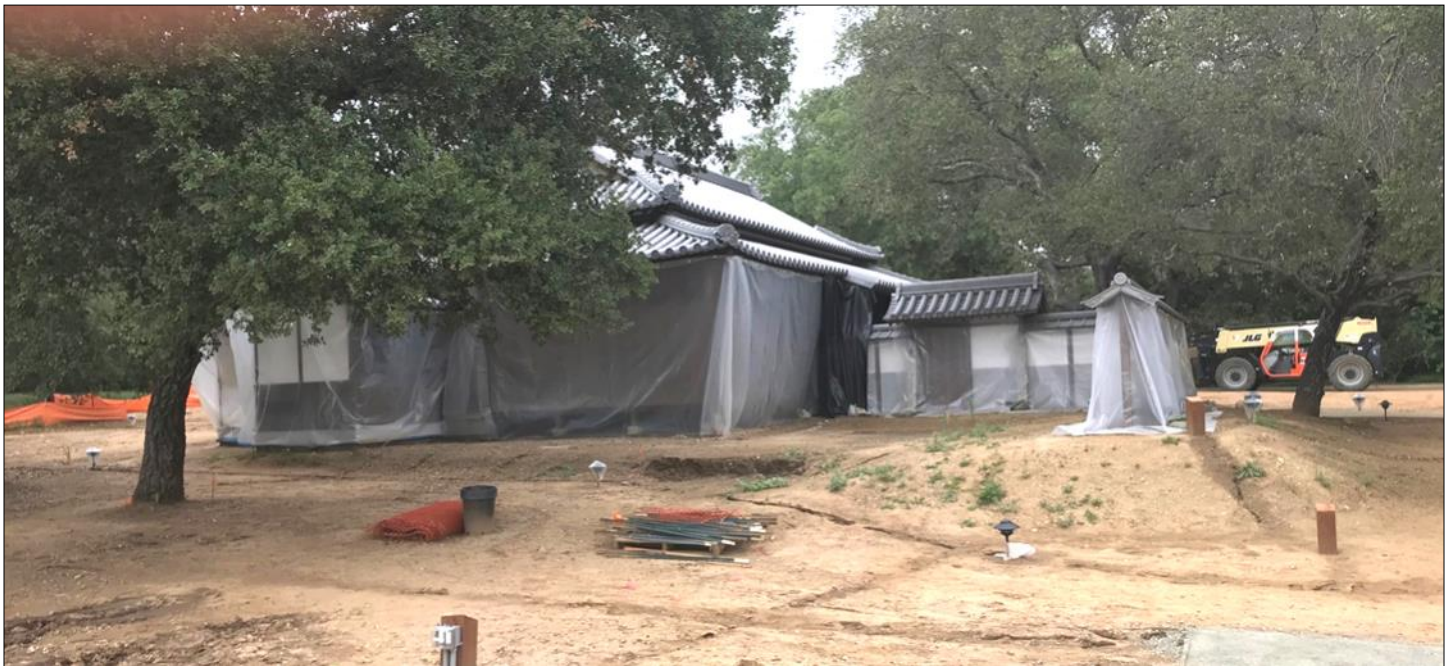
A 350-year-old Japanese farmhouse is being installed just outside the Huntington's bonsai and penjing nursery (below). Measuring a full 2,000 square feet in living space, the farmhouse was in the same family for 3 1/2 centuries before being acquired by the Huntington. It was shipped from Japan in pieces to be re-assembled here.
